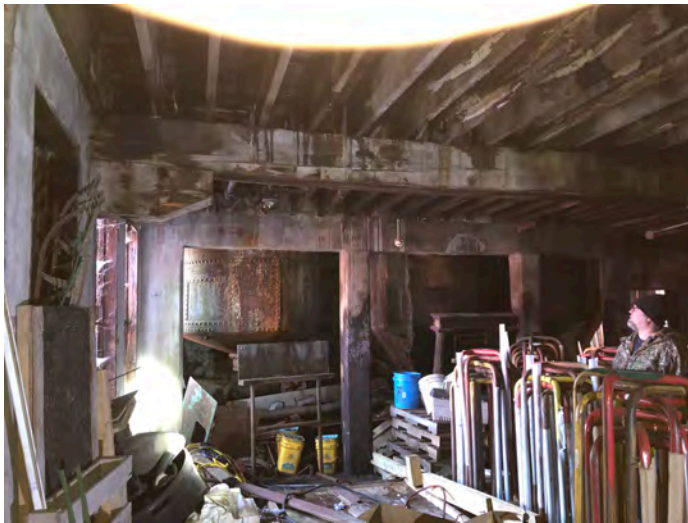
Figure 34. Back lower Level of Axle Grease looking east. -showing two tanks with concrete support posts. Photo taken January, 2023.
