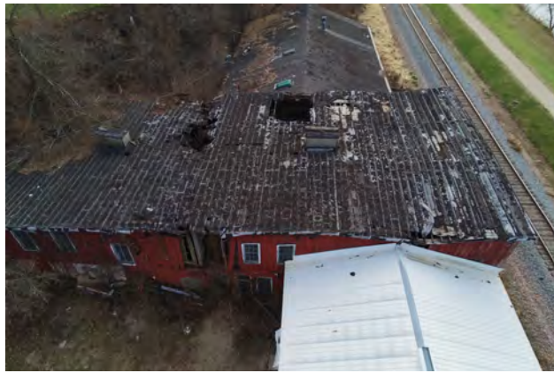
Figure 30. Aerial shot of roof of original axle grease building (middle) as of 2022. Galena Manufacturing and City of Galena building files.
