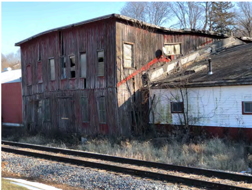
Figure 37. Galena Axle Grease building (1884) looking northeast. Building on right is 1911 addition, still in use. Photo taken January, 2023.
