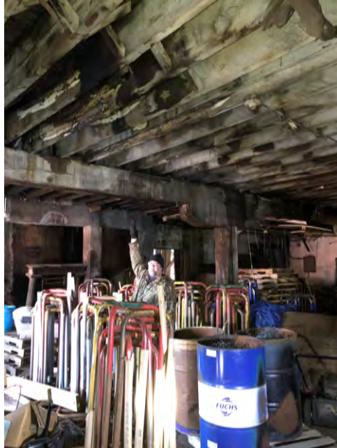
Figure 24. Original Axle Grease bldg, showing Mike Greene under deteriorated beams and joists. 1.11.2023.
