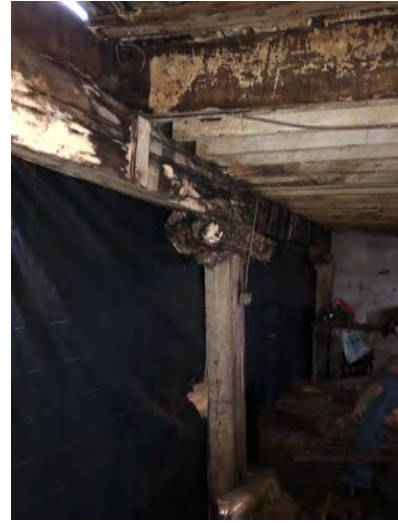
Figure 33. Axle Grease showing condition of beams and joists. Photo taken January, 2023.
