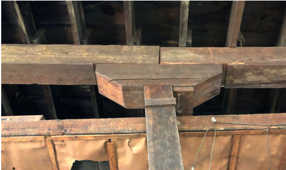
Figure 4. Axle Grease building showing construction details (one of the few sections still in good condition). January, 2023 photo.
