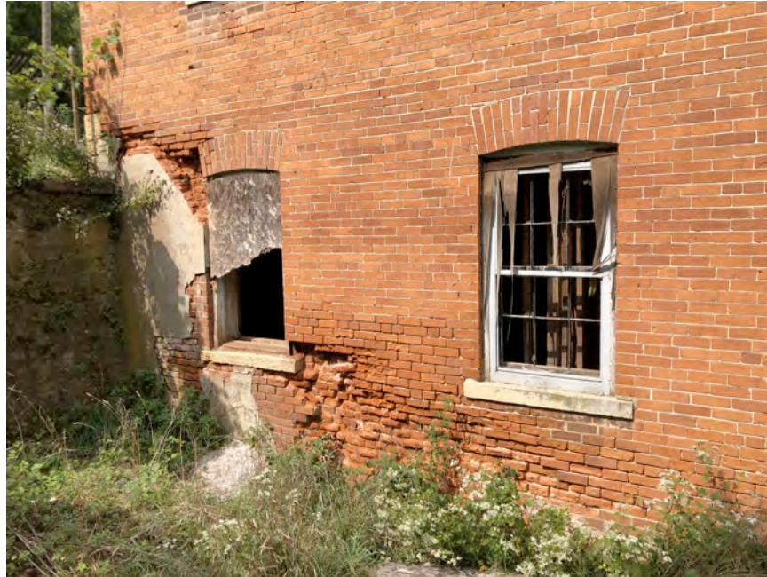
Figure 21. St. Mary's School showing deterioration of south (High St.) facade. Photo taken 14 September 2020.
