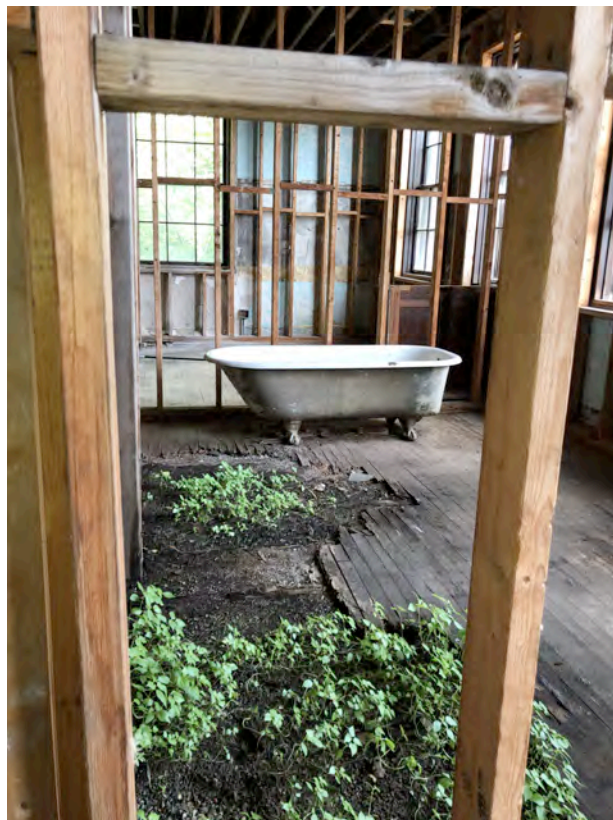
Figure 22. St. Mary's School today showing upper floor water damage from leaking roof. Also visible is the rough framing done throughout the building after all the lath, plaster and wood trim was unceremoniously removed. Perhaps the bathtub was left to catch leaking rainwater. Photo taken 14 September 2020.
