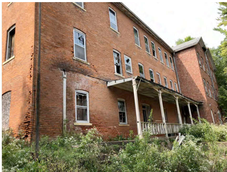
Figure 20. More years of neglect. St. Mary's School showing east facade with original 1864 section on the left. Photo taken 14 September 2020.
